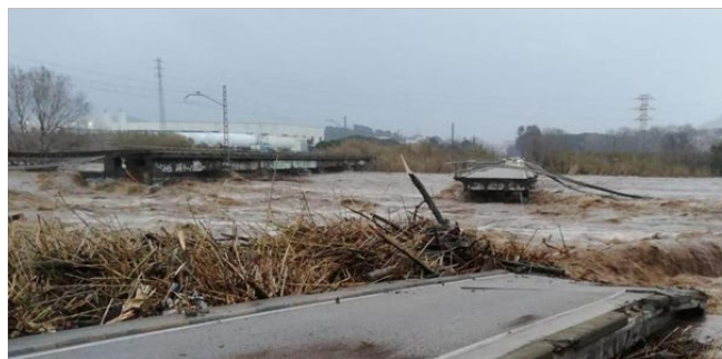
Figure 12. Damages caused by the flood in the delta of the river Tordera.
